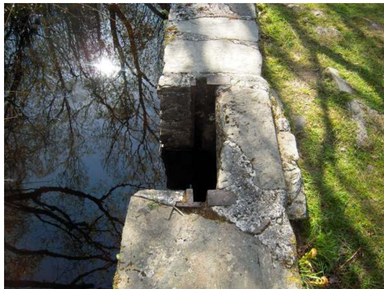
Lade sluice gate
